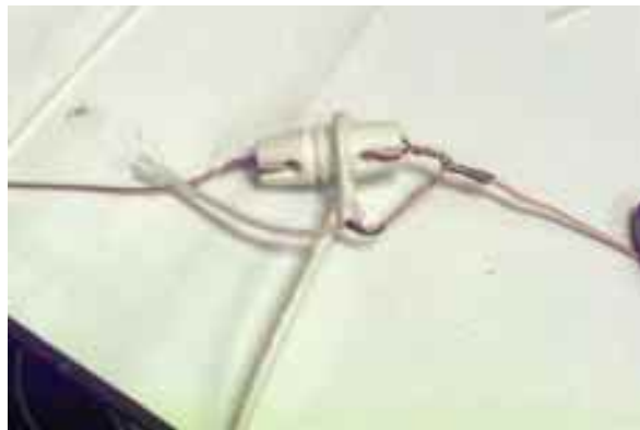
Figure 4. Tie wrap the coax over the center insulator. Wrap the center conductor around one side of the dipole and the twisted shielding around the other.
